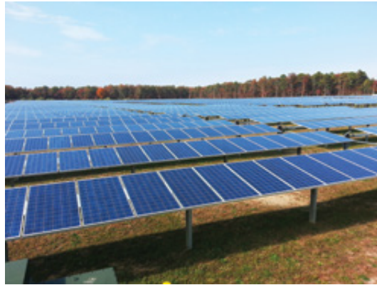
Delsea Road 3.71MW
